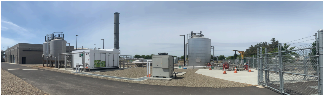
A Portion of the Water Quality Control Facility, Renewable Natural Gas Production Facility
