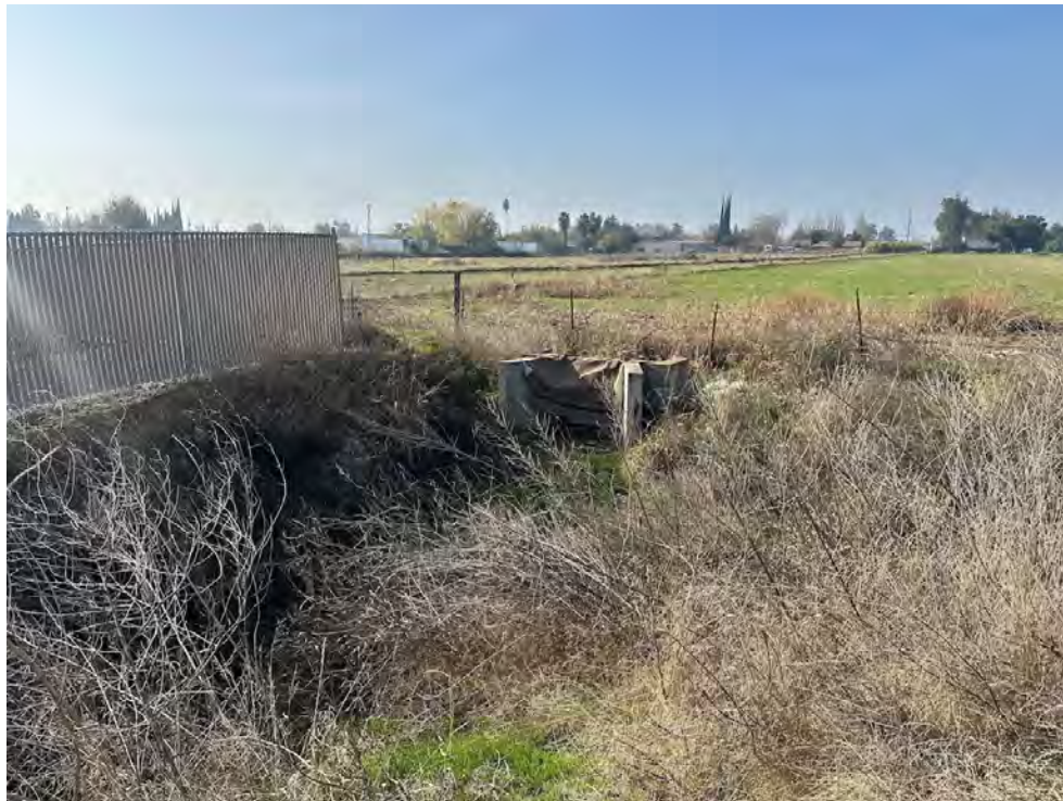
8. Facing west, the photo shows the culvert, located outside of the Survey Area, where water from feature ED 1b flows underground into the stormwater drainage system.
